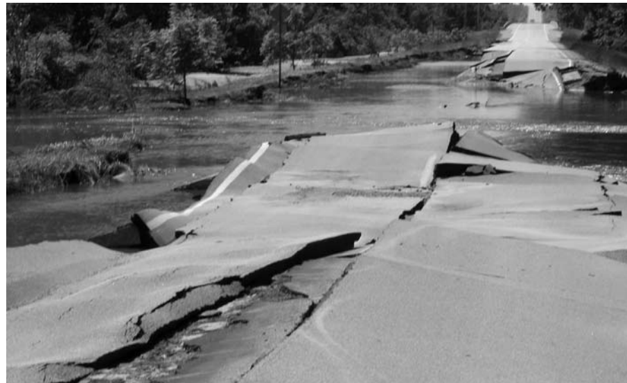
Flood damage disrupted transportation over a wide area of Iowa.
