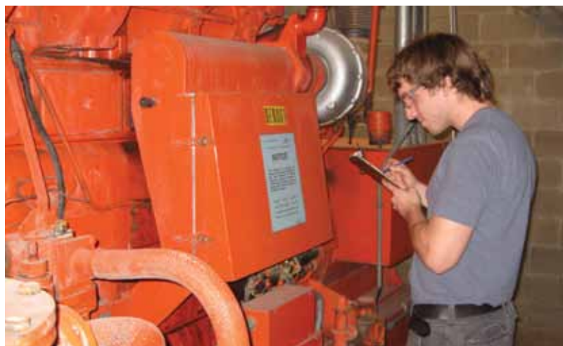
Top: Kevin Mann, junior in mechanical engineering, checks the nameplate specifications on an electric motor and pump. Bottom: Industrial engineering senior Ryan Frahm checks the nameplate ratings of a backup generator.
